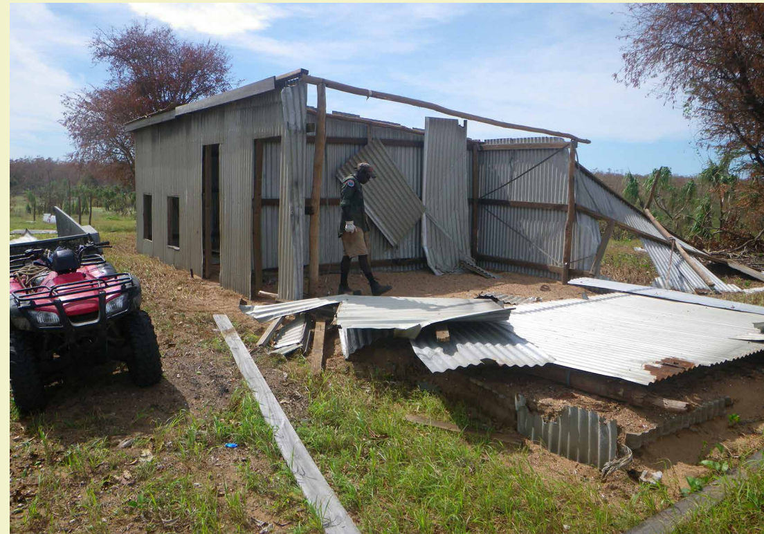
A Crocodile Islands Ranger helps repair cyclone damage at Mooroongga. Photo © Crocodile Islands Rangers
